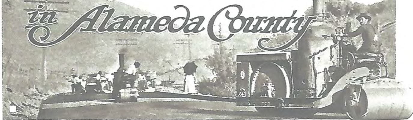
Putting the finishing touches on a new section of road in Bulmer Hill cut.
